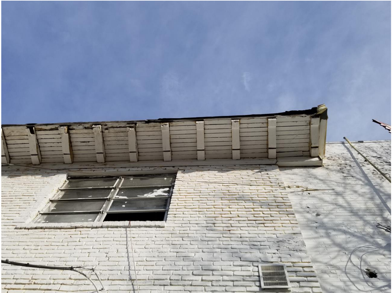
#17 – Middle portion of left side (west – Argonne Ave, NE) façade and eave detail, looking up
