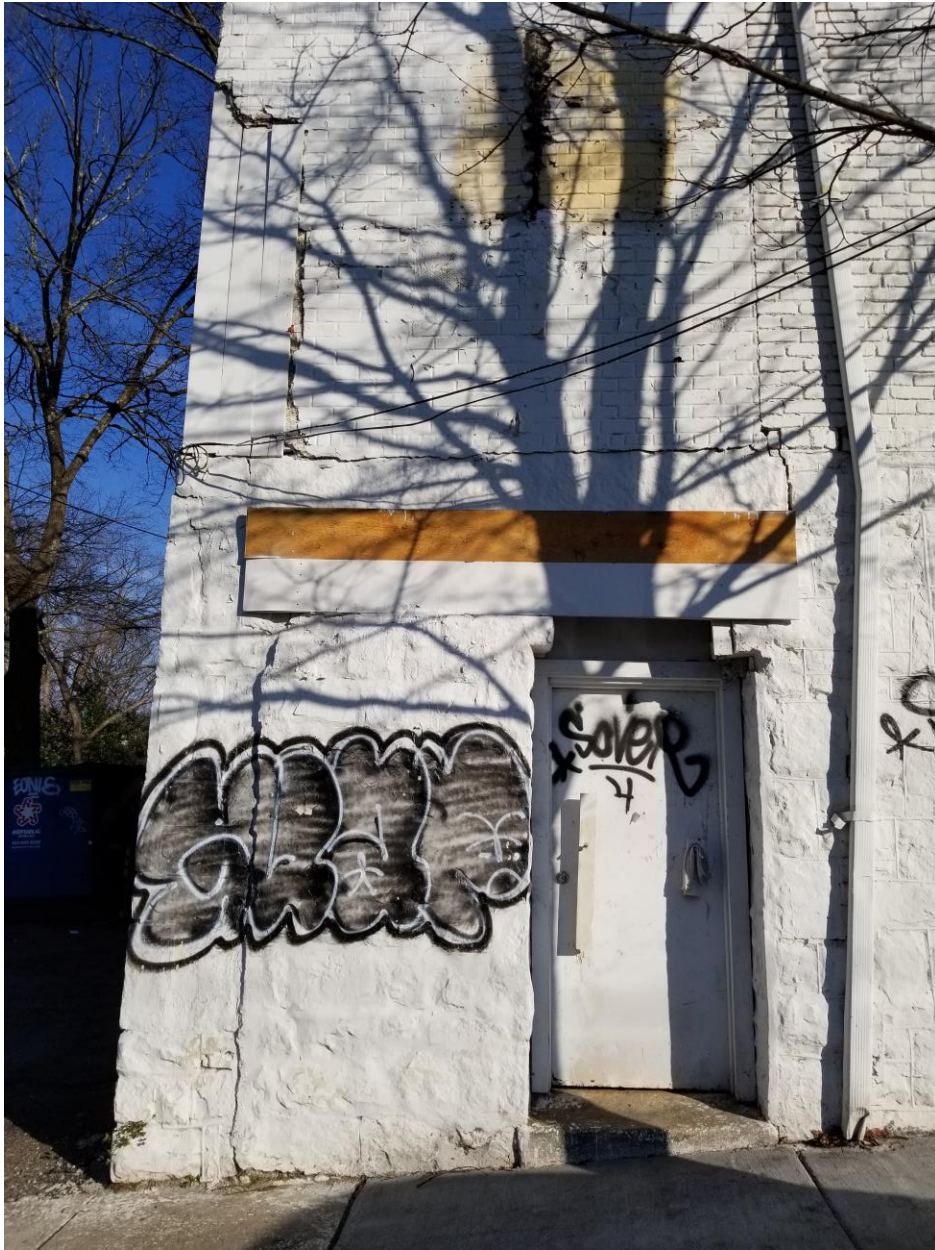
#14 – Rear portion of left side (west - Argonne Ave, NE) façade, looking east
