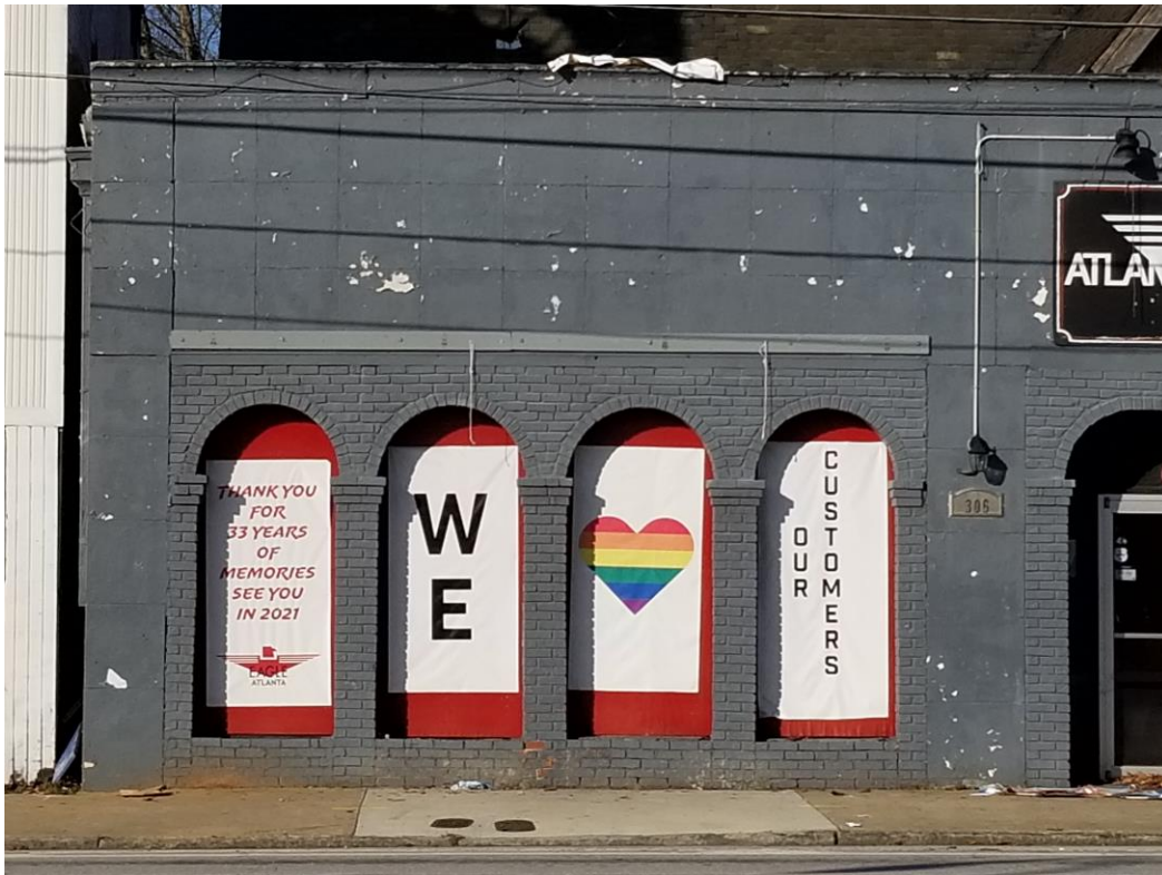
#4 – Lower west portion of front (south – Ponce de Leon Ave, NE) façade, looking north
